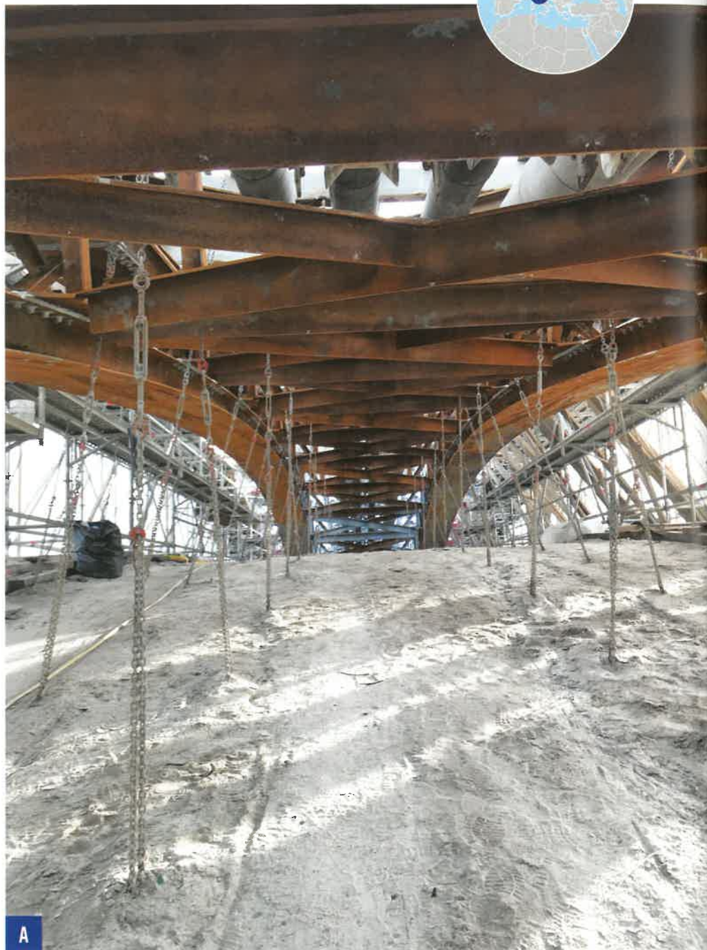
A: The underside of the Academia Bridge. B: The steel water pipe system. C: Venice's historic Academia Bridge. D: Relining taking place within the host pipe.
